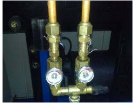
An example of good practice in pipework
